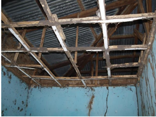
Ceiling affected by termites and
